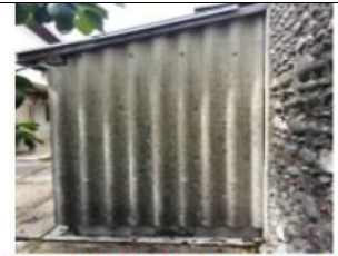
PLAQUES FIBRES CIMENT AMIANTES
