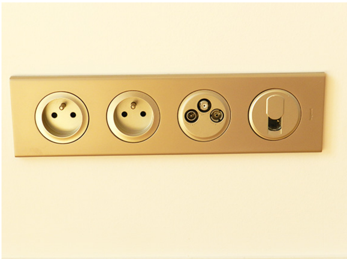
Typical Sockets:- Power / TV / Cat 5e
